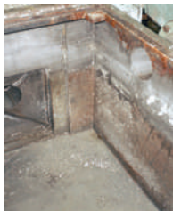
Corrosion in the reservoir
